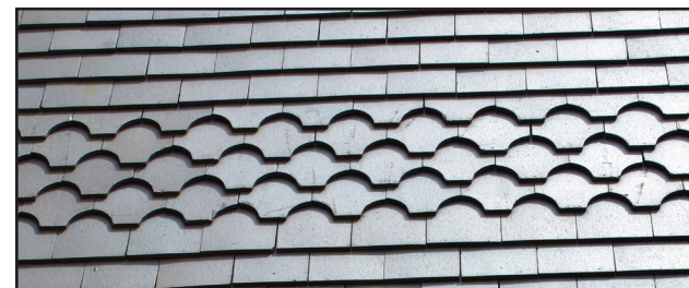
Figure 21 Decorative slates on St Mary's roof, recently replaced and referencing the nineteenth century design.
